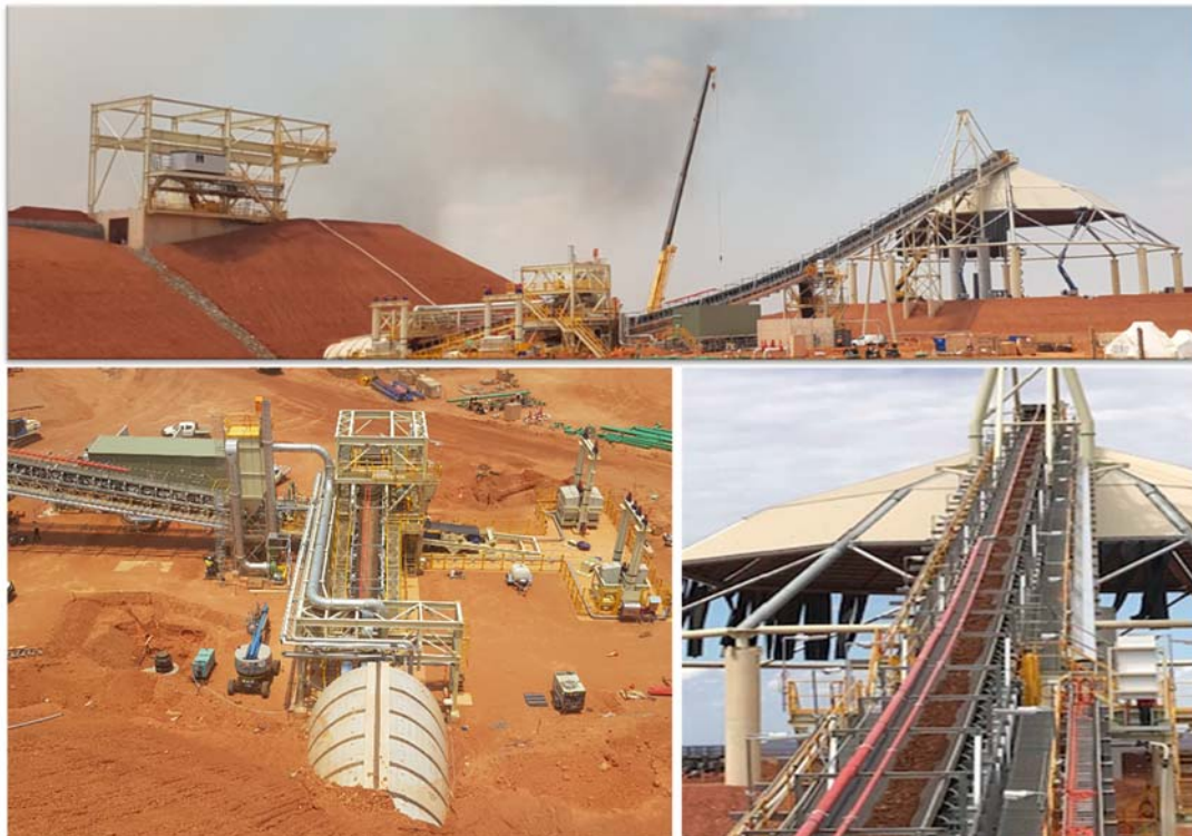
Photos clockwise from top: primary crusher to coarse ore stockpile circuit, CV02 delivering material to the coarse ore stockpile, CV01 transfer station to CV02
