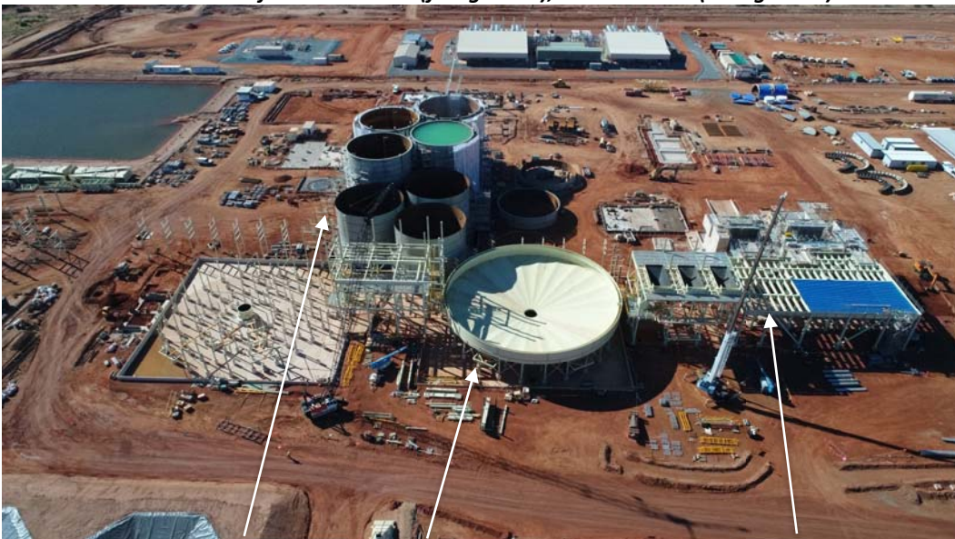
Aerial view of CIL tanks, pre-leach thickener and base structure for the SAG and Ball Mills
